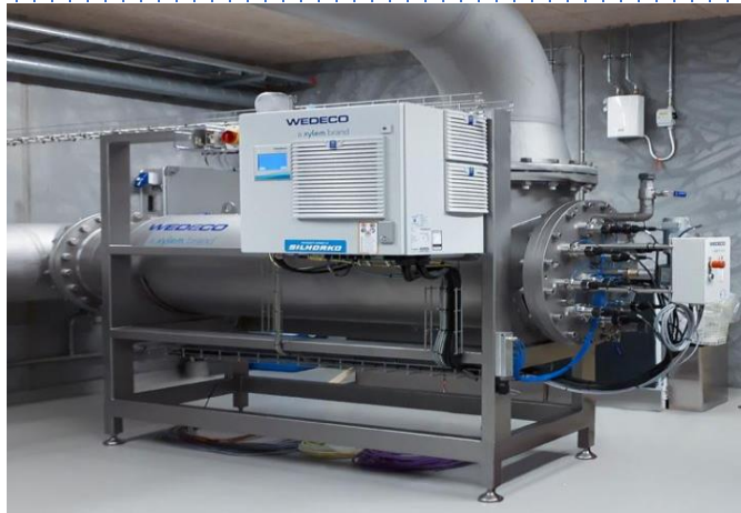
Ultraviolet water disinfection system
