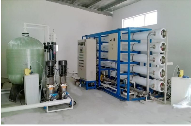
Pic.2 Reverse Osmosis Cleaning Equipment
